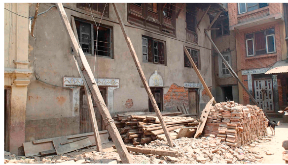
Fig. 3. Example of historic building in Patan damaged by the earthquakes and supported by wooden braces. (Photo P. Daly).
